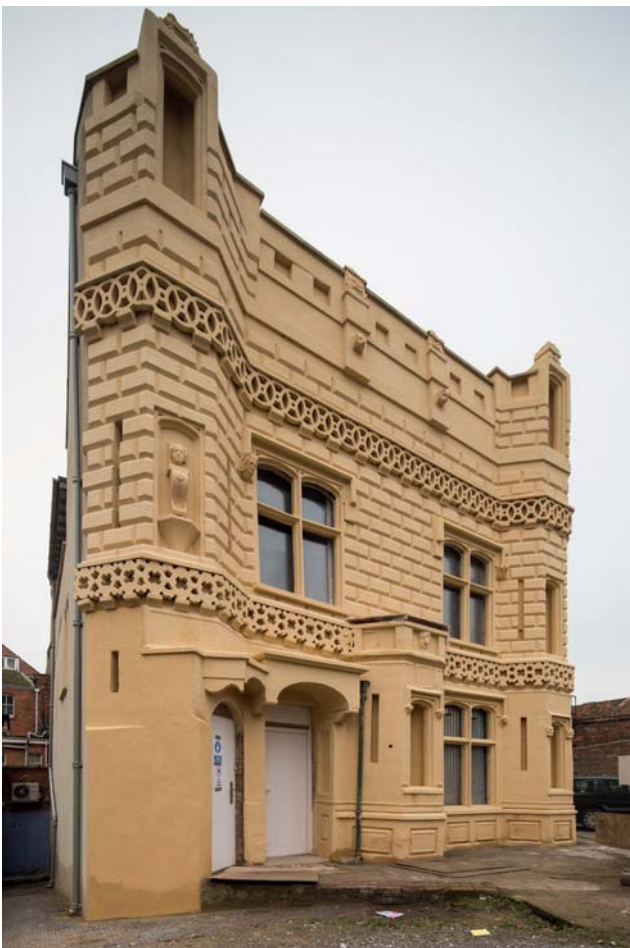
The restoration of the façade of Castle House in Bridgwater in Somerset is now complete showing decorative concrete details including gargoyles (image: Eveleigh Photography)
