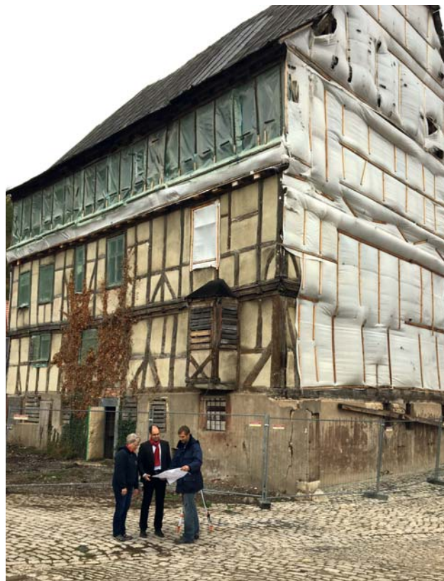
The Hessischer Hof is an imposing timber structure in the town of Treffurt in Germany (image: Stadt Treffurt)
