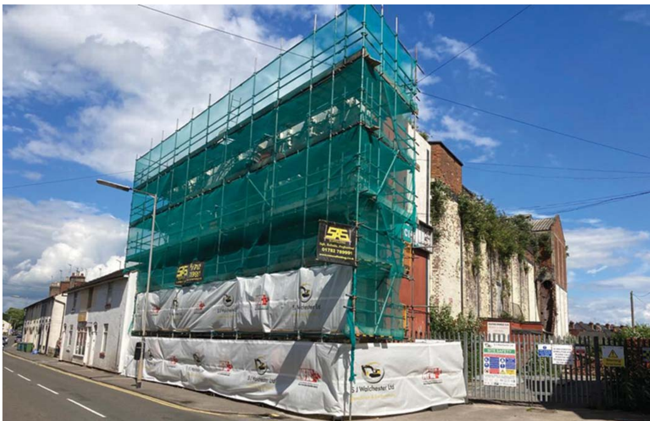
The Sandonia was scaffolded on the day demolition began illegally in July 2021 (Credit: Save Our Sandonia)
