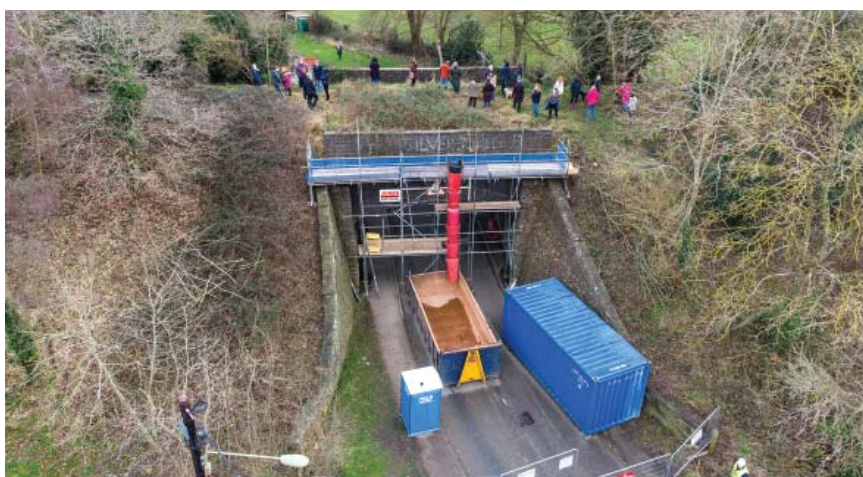
Villagers gathered on a bridge at Horspath, Oxford, after a National Highways contractor started to demolish its parapets (Credit: The HRE Group)
