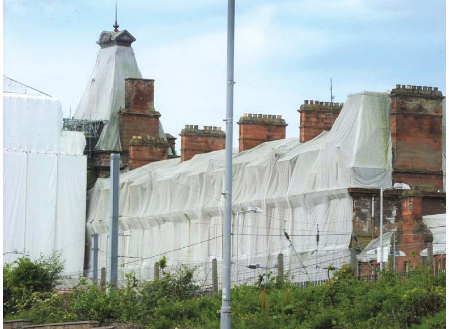
The station hotel has been hidden under protective scaffolding since 2018 (Credit: Ayrshire Post)
